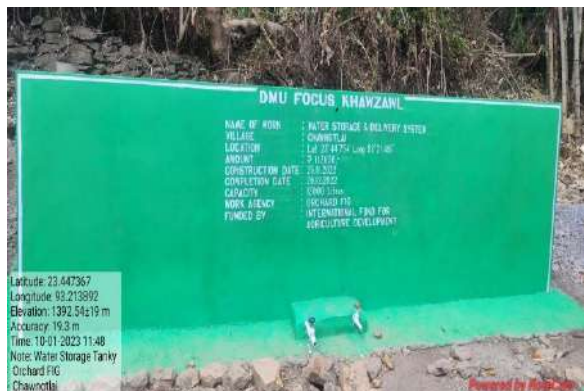
Water Storage & Delivery System
