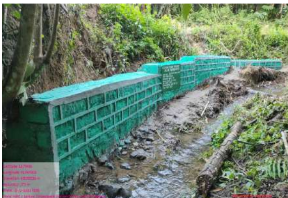
Stream Bank Erosion Control
